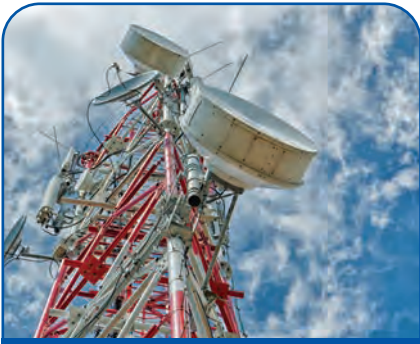
Telecom -Data Infrastructure
